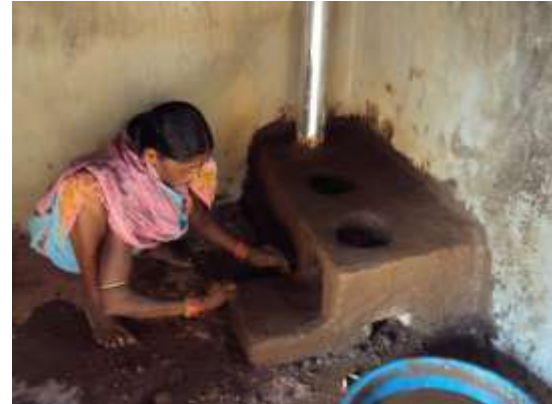
Installation of smokeless wood efficient stoves
